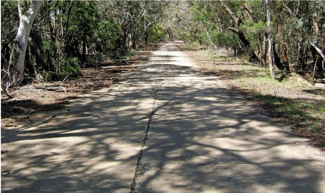
Figure 1: Sydney - Melbourne Highway approximately 200km south west from Sydney (Marulan) constructed 1927. This pavement was in service until the early 1980s before a major realignment of the highway
