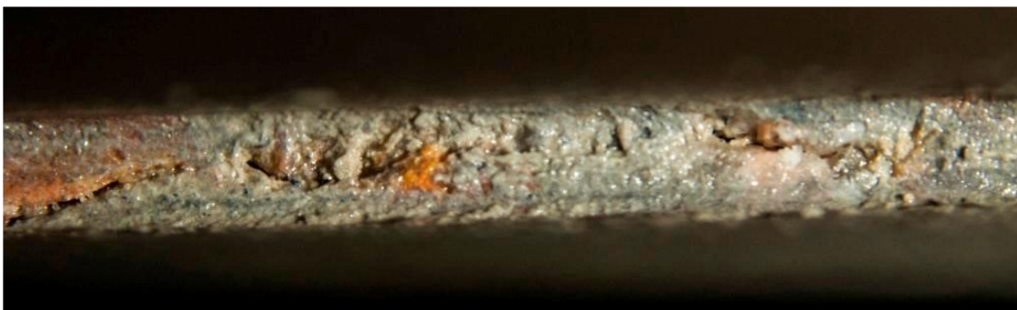
Figure 21: (a) Specialised photography looking down into sawcut confirming induced longitudinal crack at base of sawcut
